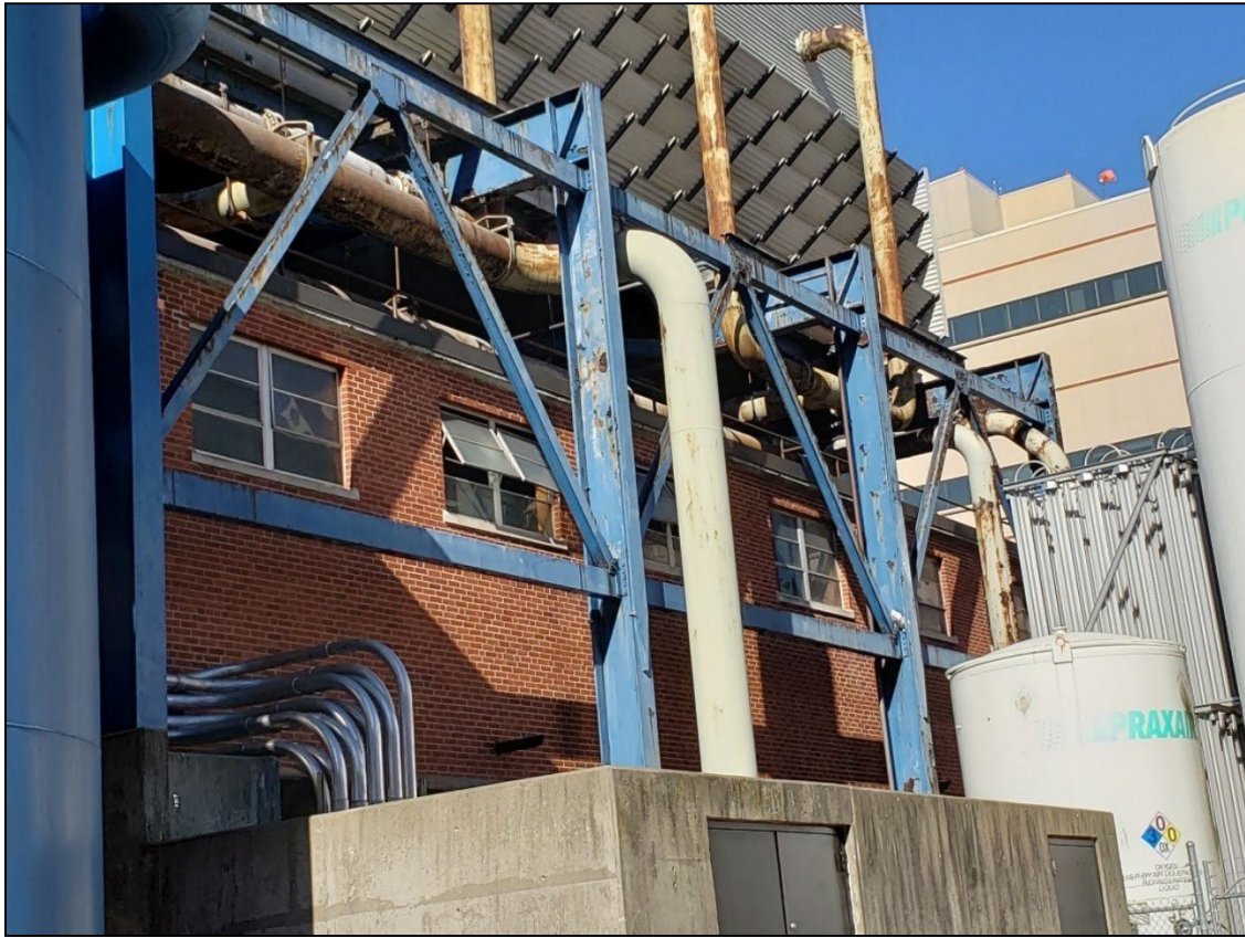
Photo 001 Overview of Northeast Face of Structure Rust and spalling paint were observed at the four exposed columns and vertical lateral braces. They mainly occurred on the face of the column webs and brace flanges.
