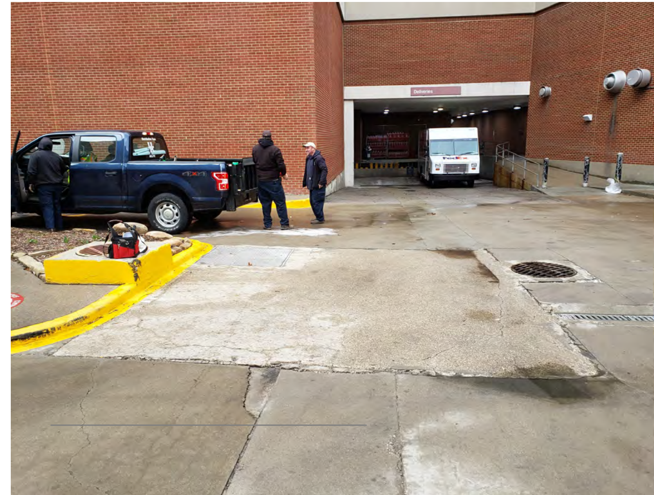
VIEW OF TOP SLAB OF EXISTING VAULT CRACKS AND STANDING WATER WERE OBSERVED AT THE TOP OF THE EXISTING VAULT.
