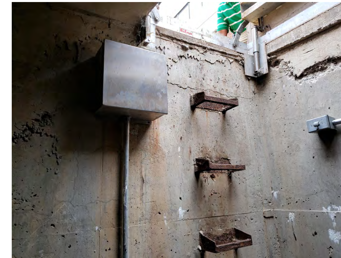
VIEW OF MANHOLE ACCESS OF EXISTING VAULT CRACKS AND SPALLING CONCRETE WERE OBSERVED AT THE WALL SURFACE OF THE EXISTING VAULT AT MANHOLE ACCESS.
